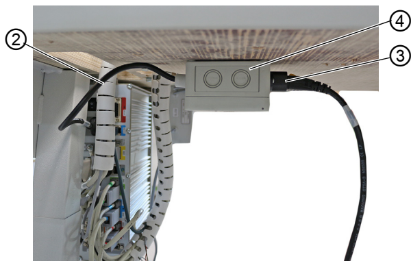
(2) - Cable (3) - Power cable
